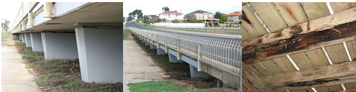
Figure 8 Bridge Condition Example: 1, 4, 9 from left to right
