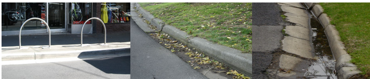
Figure 7 Kerb Condition Example: 1, 5, 9 left to right
