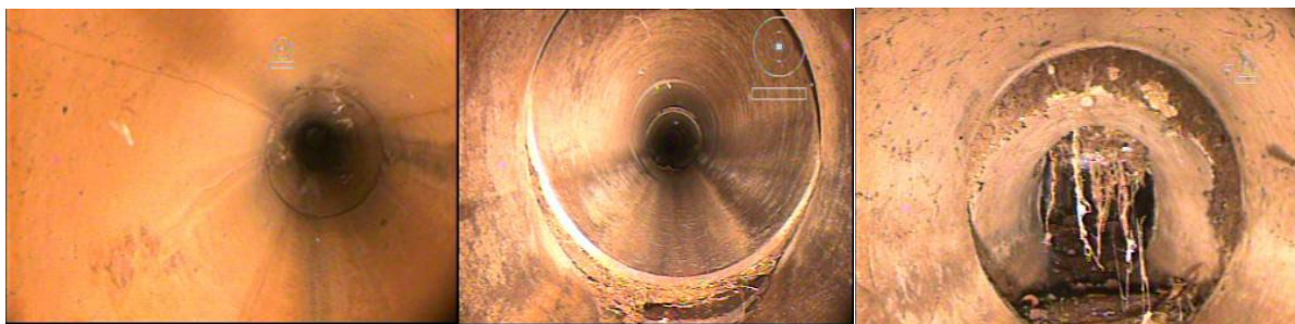
Figure 16 Pipe Condition Example: 2, 5, 8 from left to right
