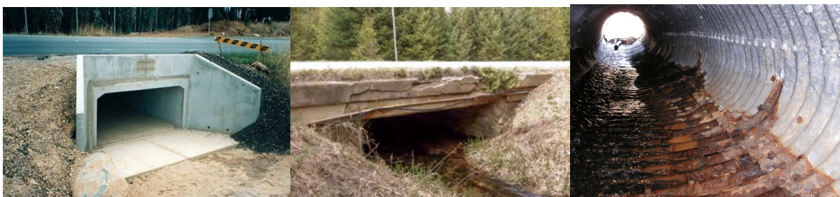
Figure 10 Culverts Condition Example: 1, 5, 7 from left to right
