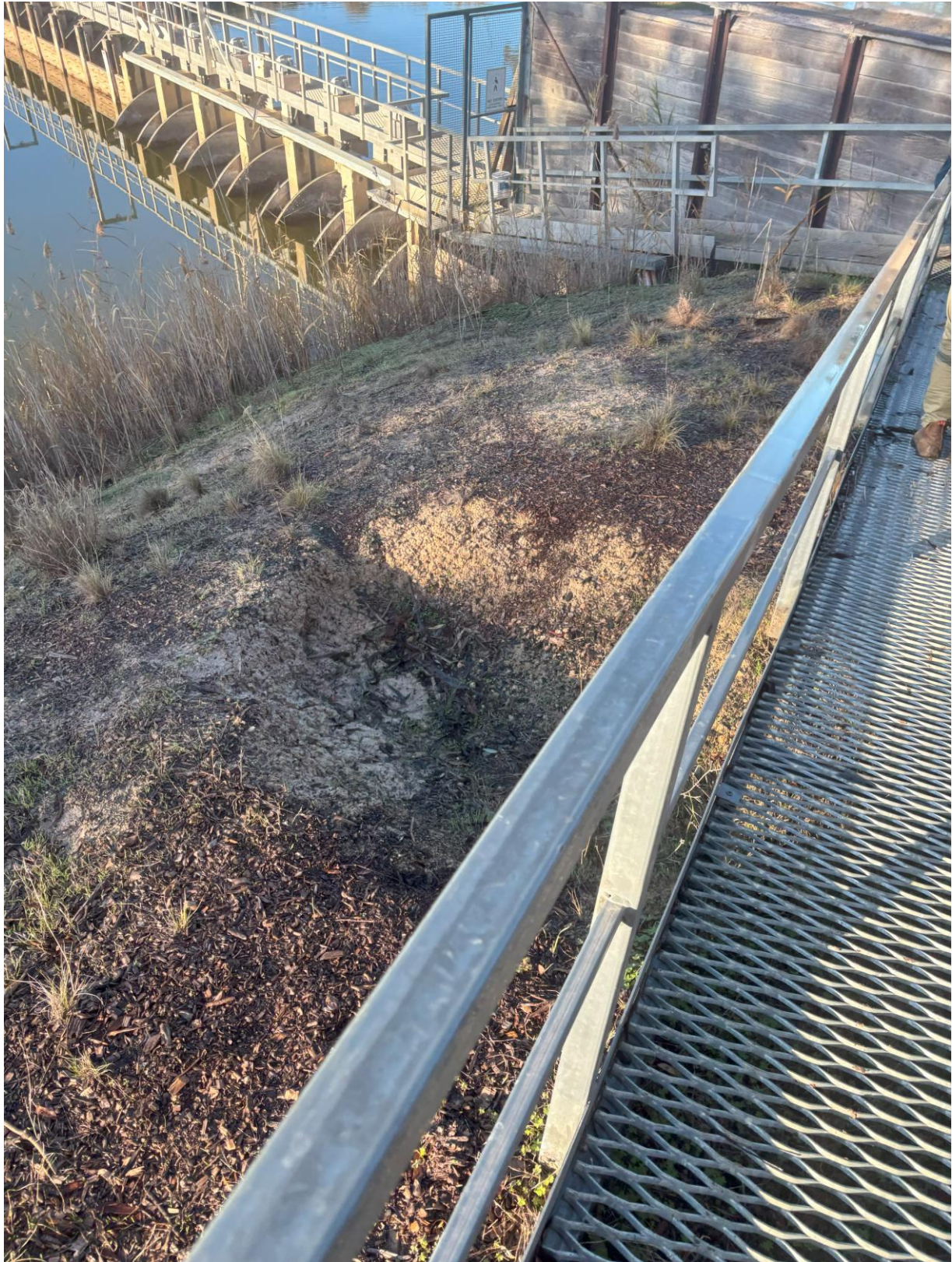
Photograph 10 – Continuation of the erosion along the entry fence line.
