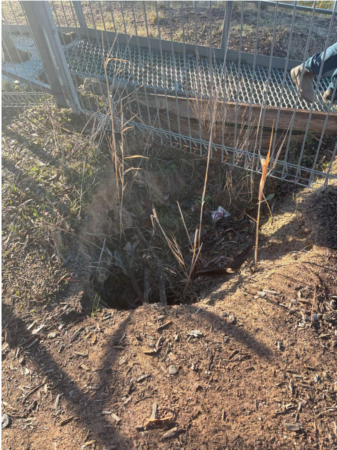
Photograph 9 – Erosion along the entry fence line.
