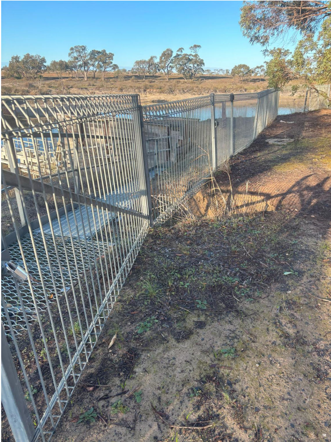
Photograph 5 – Erosion along entry fence line
