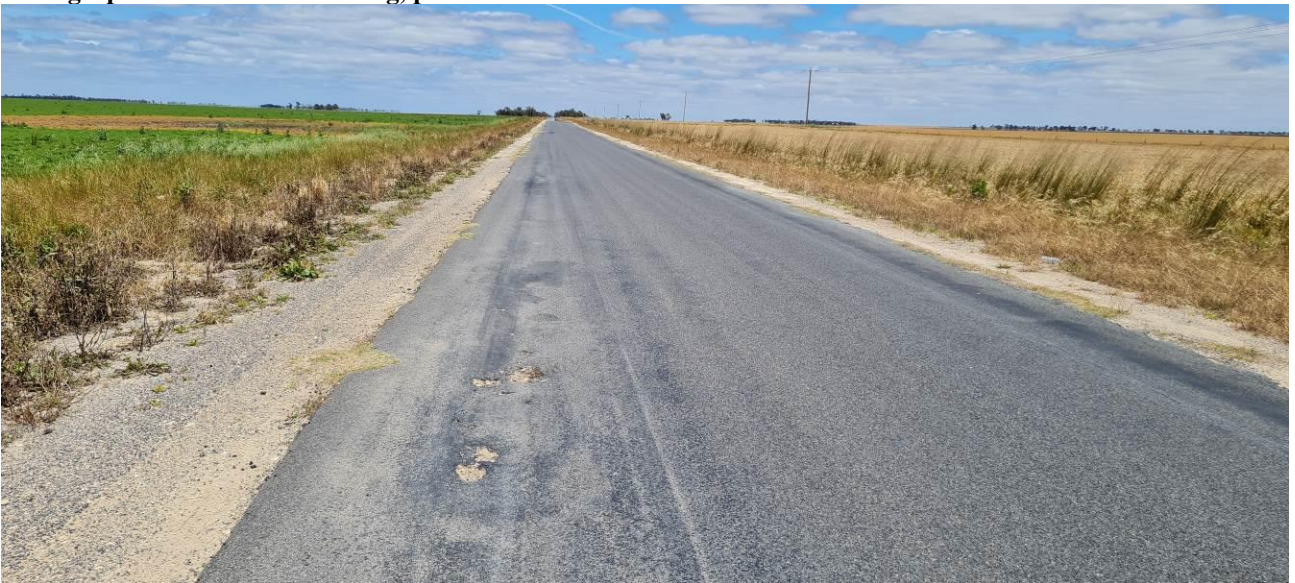
Photograph 17 - Ch 6.8 Potholing and deformed pavement
