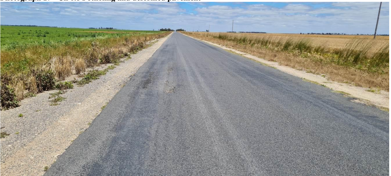
Photograph 18 - Ch 6.85 Seal breaking up and potholing
