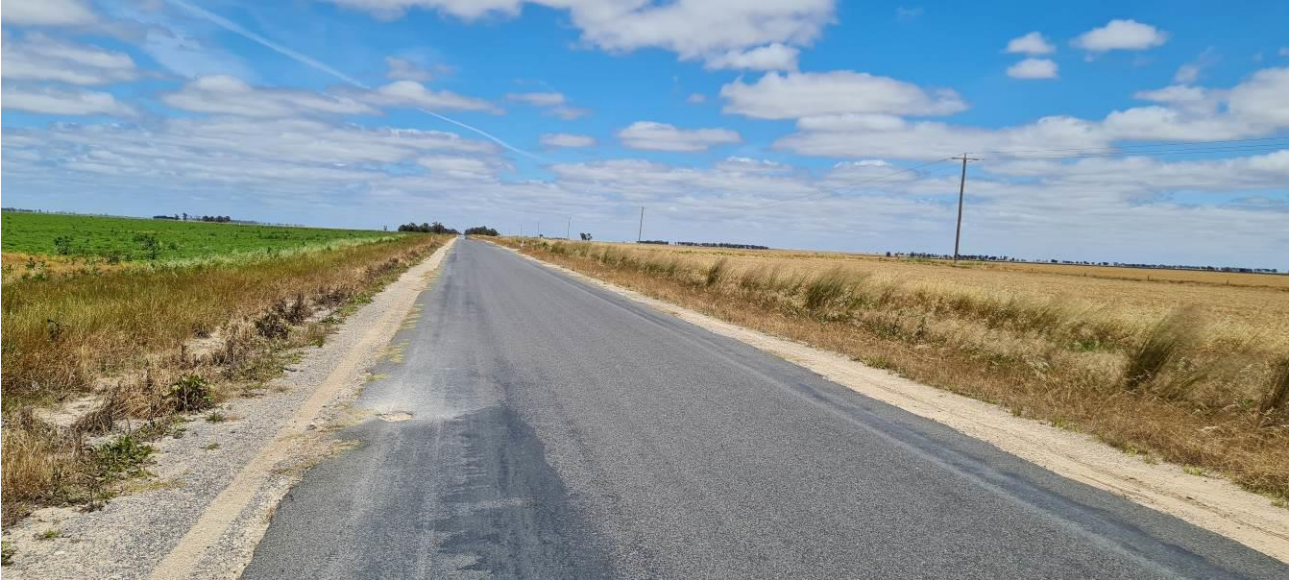
Photograph 16 – Ch 6.75 Potholing, polished and deformed seal
