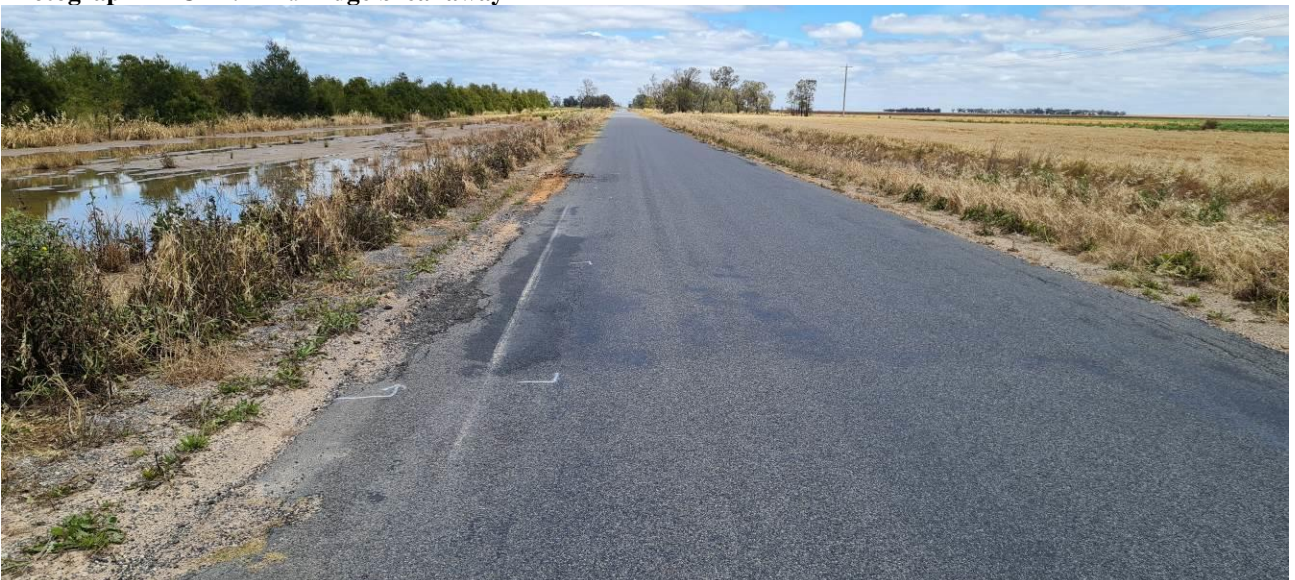
Photograph 3 - Ch 5.4 - 5.6 Edge breakaway and shoving
