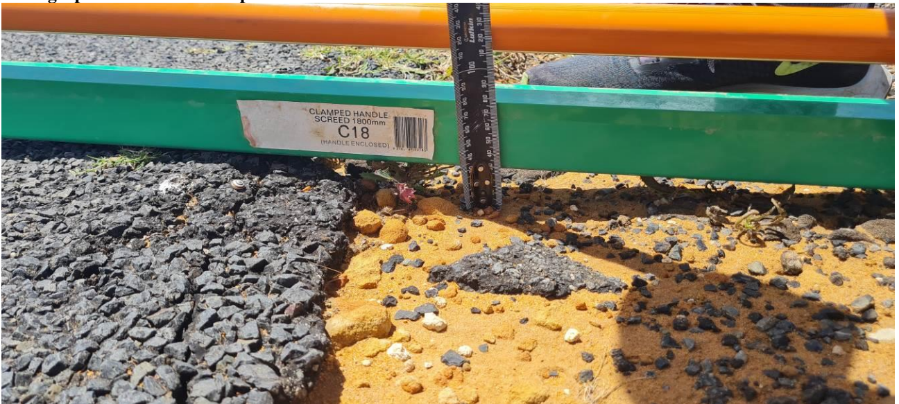
Photograph 48 - Southern drop off 30mm
