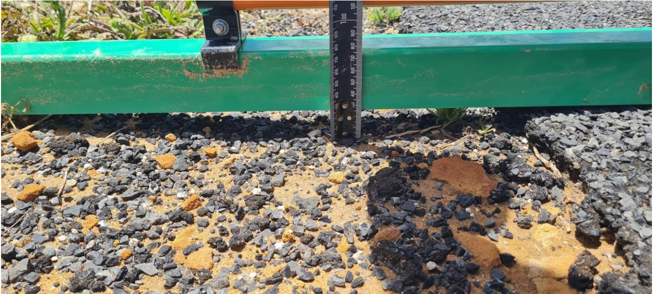
Photograph 47 - Northern drop off 36mm
