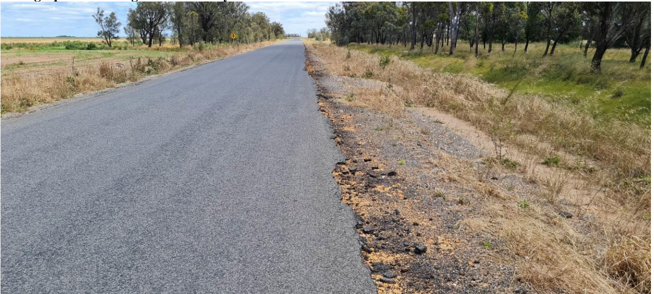
Photograph 2 - Ch 4.7 - 4.9 Edge breakaway
